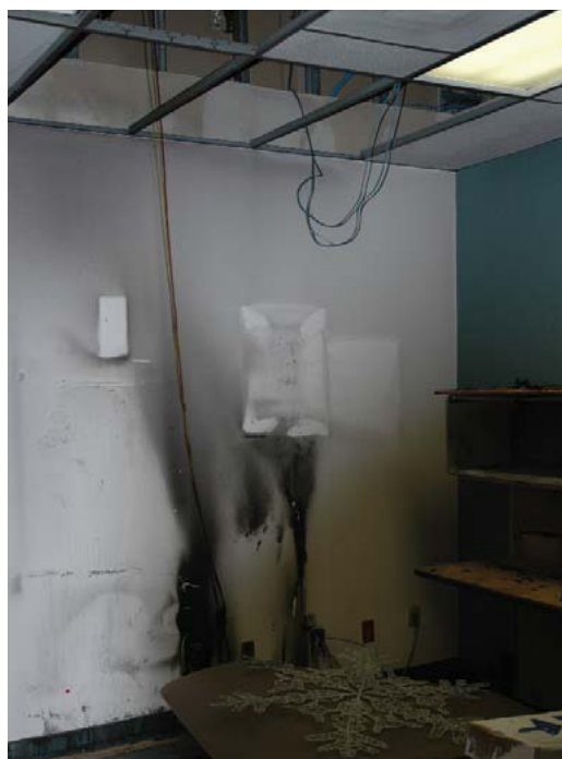
An interior office with evidence of smoke damage on the walls. Photo credit: Randy Silverman
